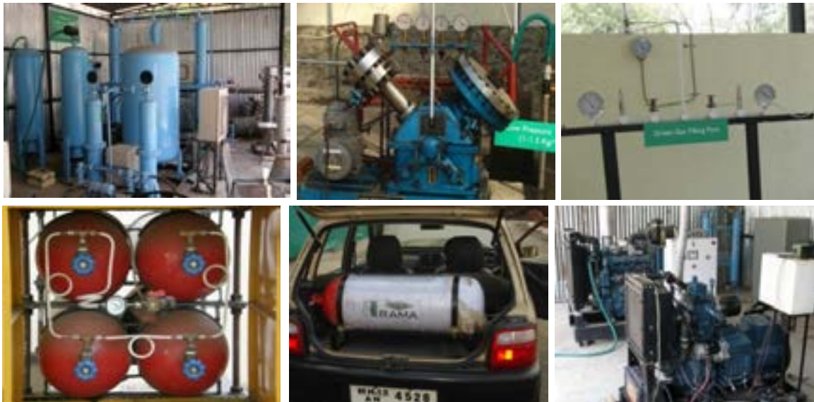
EXPERIMENTAL SETUP FOR BIOGAS TO FUEL (SCRUBBER, COMPRESSOR, STORAGE, DISPENSING TO USE) AND BIOGAS TO POWER (GENSET)
